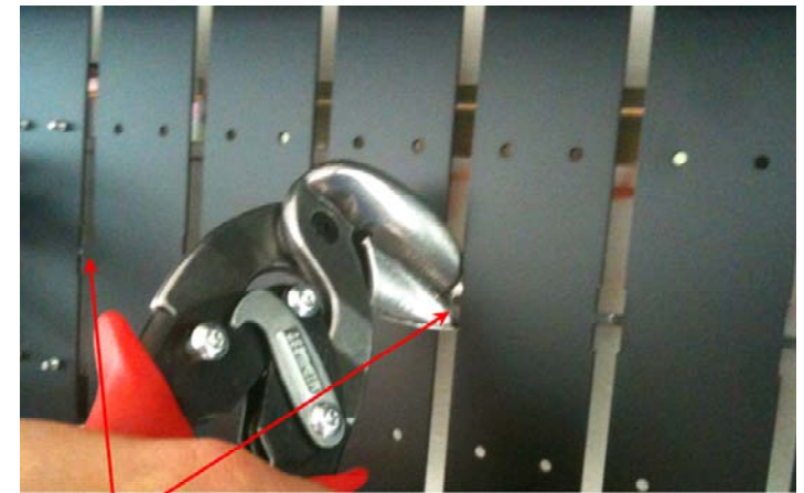
Tabs to cut to allow ticker to flex to follow the curve of a wall.
